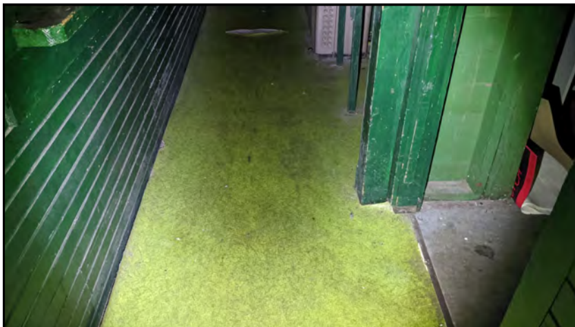
PHOTO 34 Floor linoleum flooring and paint in common area.
