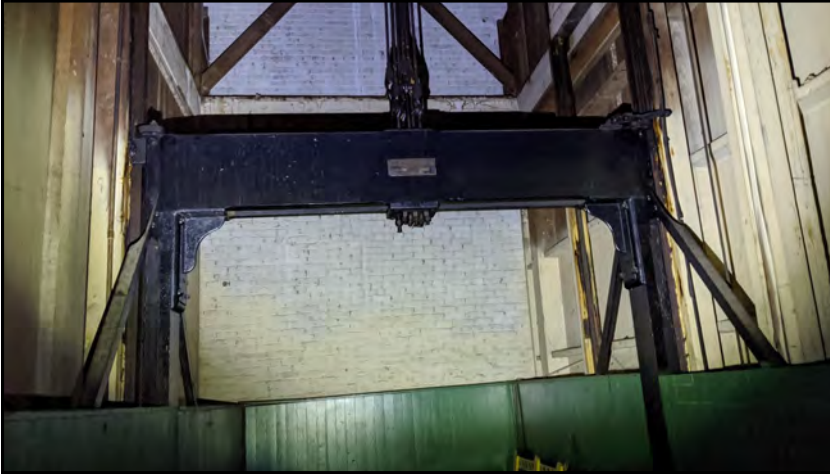
PHOTO 28 Cable operated freight elevator.
