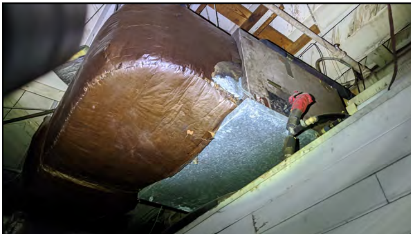
PHOTO 31 Duct insulation in former bottling plant.
