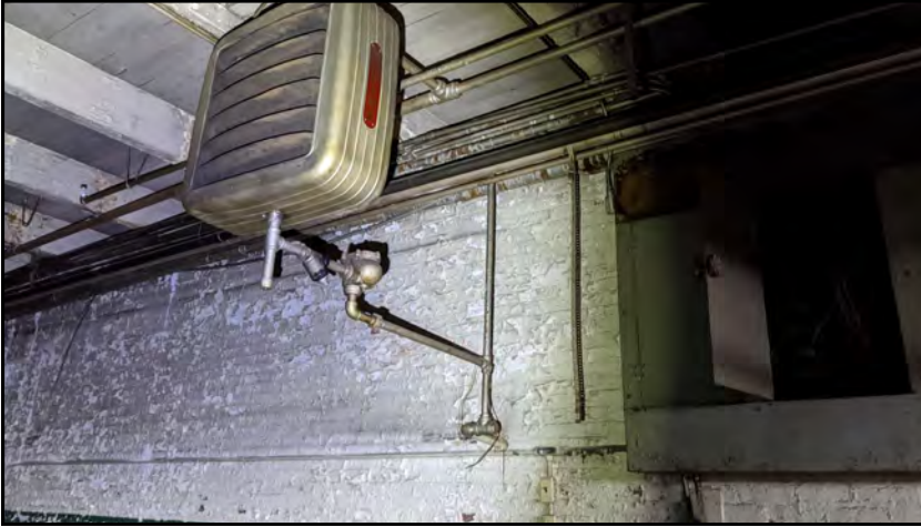
PHOTO 43 Heater unit in production area.
