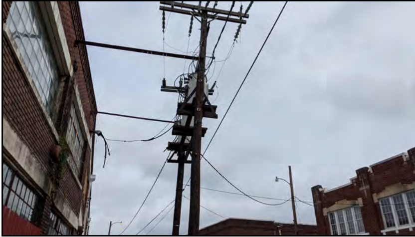
PHOTO 7 Pole-mounted electric transformers on the east side of the subject property.
