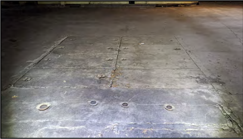
PHOTO 22 Scarring in concrete of stor- age area.
