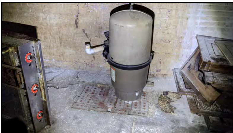
PHOTO 27 Water filtration and floor drain in bottling factory.
